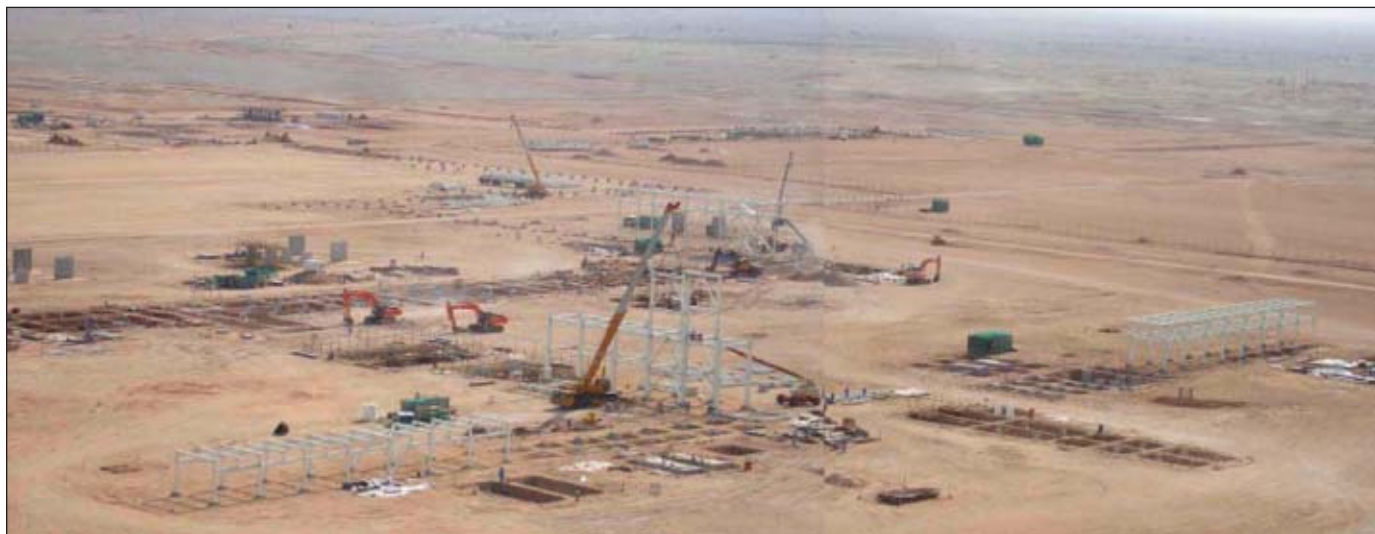
Miscible sour-gas injection facilities are under construction for the Harweel cluster (Fig. 6). Photo from PDO.
