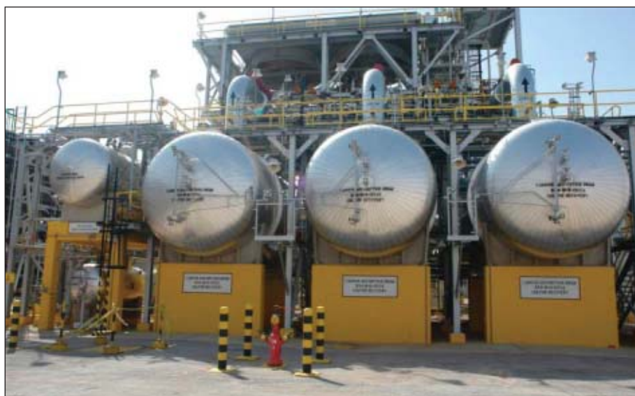
This is one of the seven carbon-bed BTX-removal units (Fig. 1).
