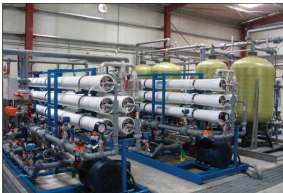
A reverse-osmosis process lowers the total dissolved solids in feed water going to the steam generators at Amal West (Fig. 3). Photo by Guntis Moritis.
