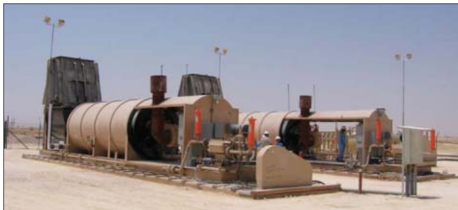
Two, 200 ton/day, skid-mounted steam generators produce the injected steam in the Amal West pilot (Fig. 4). Photo by Guntis Moritis.
